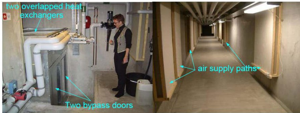
Figure 2.13: Air distribution duct of Mediã school (Left photo shows heat exchangers and “summer” doors. Right photo shows the supply air paths) (Paolo and Roberto, 2009).
